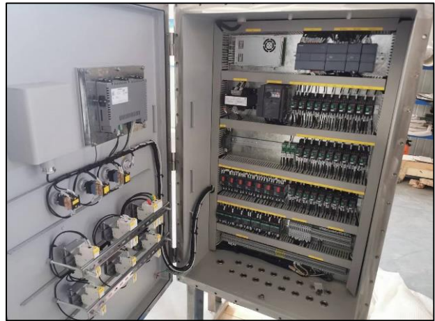
Inside the explosion-proof electric cabinet
